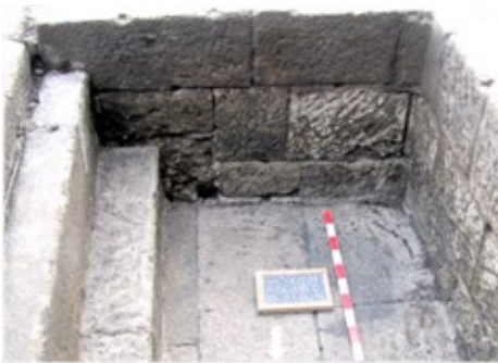
Figure 4: Opus caementicium substratum visible at the bottom of the steps of pool D.
